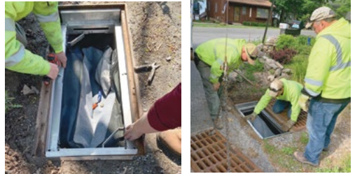
Frankford Township DEP employees installing insert protection bags supplied by the GCLWCF.
